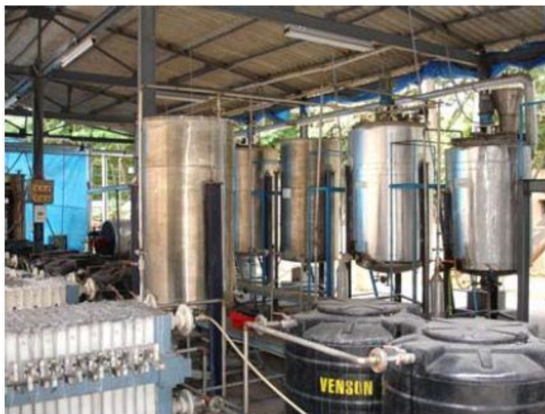
Figure 2. A pilot plant for rice husk incineration in India [38]
